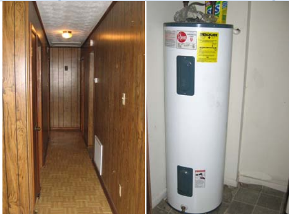
Paneled hallway connecting the three bedrooms, bath and laundry areas. Electric water heater is only __ years old.
